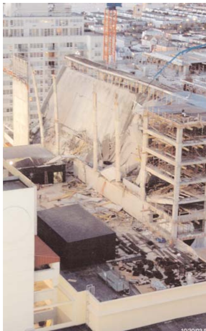
Tropicana Parking Garage Collapse
